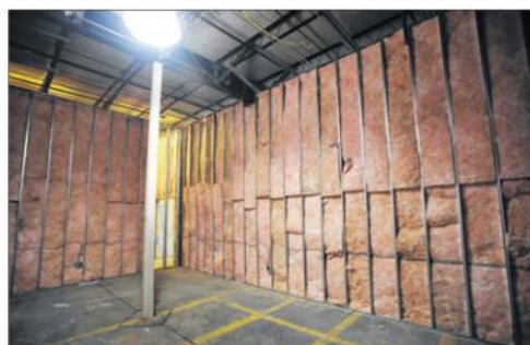
Production Manager Klaus Poltila, left, and Managing Partner David Lipton at the Advanced Grow Labs medical marijuana growing facility being constructed at 400 Frontage Road in West Haven.
